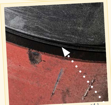
• exposed threads susceptible to corrosion
